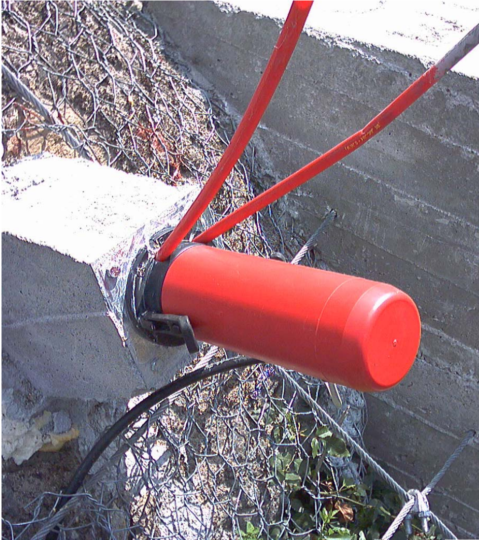
MPBX on dam abutment
